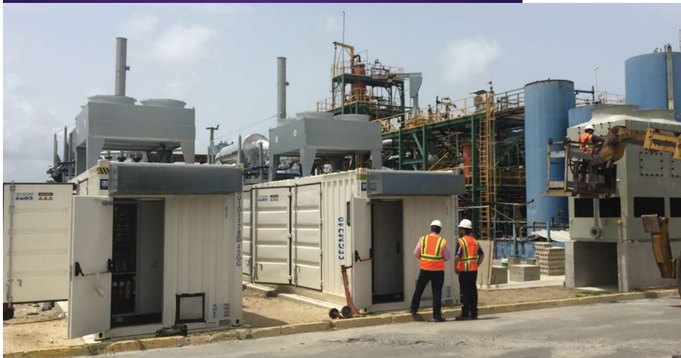
Olein food industry plant, two containerized SGE-24SM engines.
