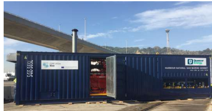
Containerized 56SL genset for harbour use.
