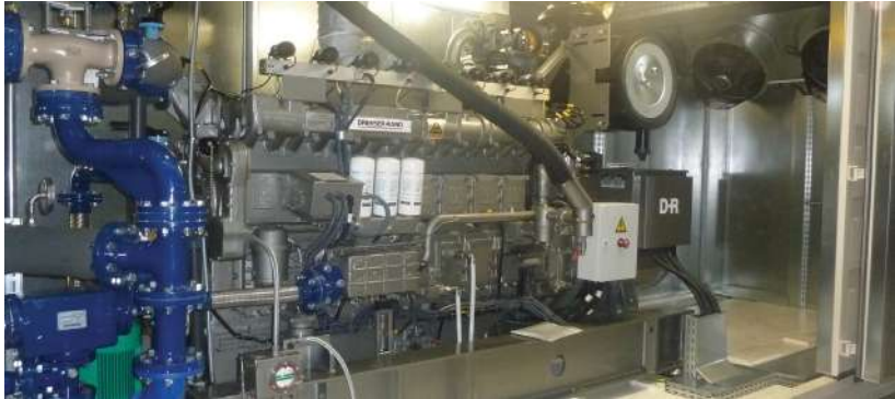
A CHP package of SM genset.
